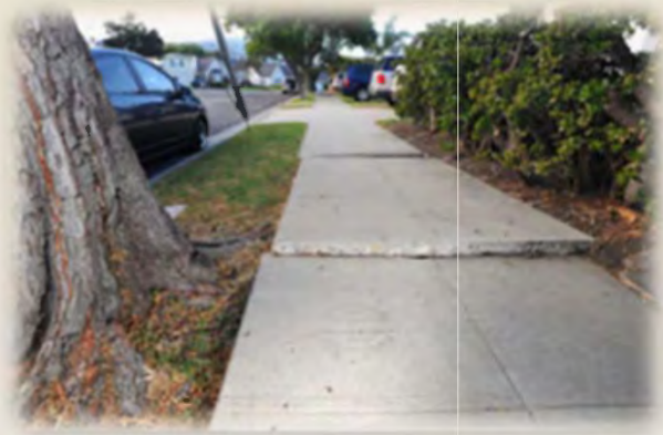
TREE ROOTS— #1 Cause for lifted sidewalks
